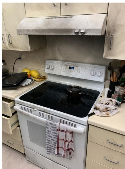
Stove top cooking fire damage
