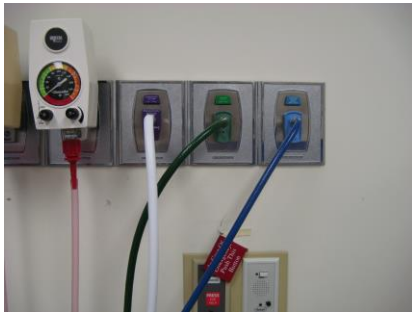
Image 1: Gas lines from wall in dental office/clinic
